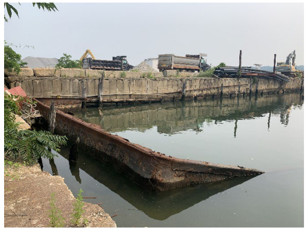
Sunken barge visible adjacent to the concrete bulkhead.
