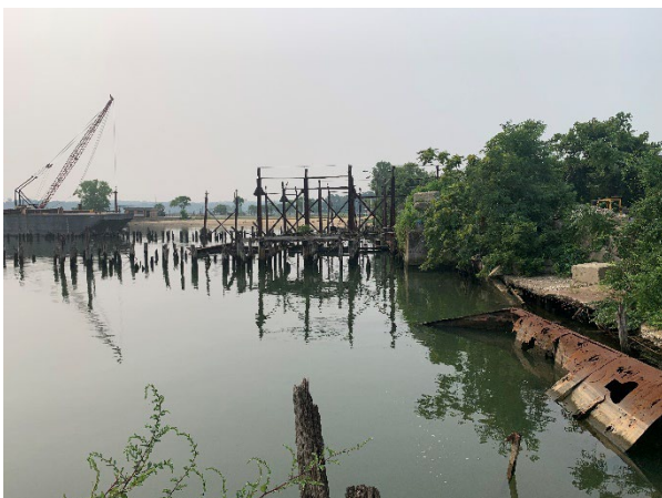
View of the dilapidated steel dry dock and remaining piles of the former timber pier, facing south.
