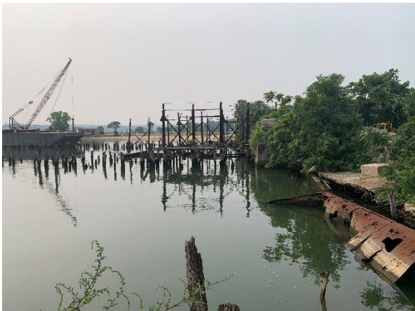
Deteriorated timber and steel structures visible at the underwater portions of the Subject Property.
